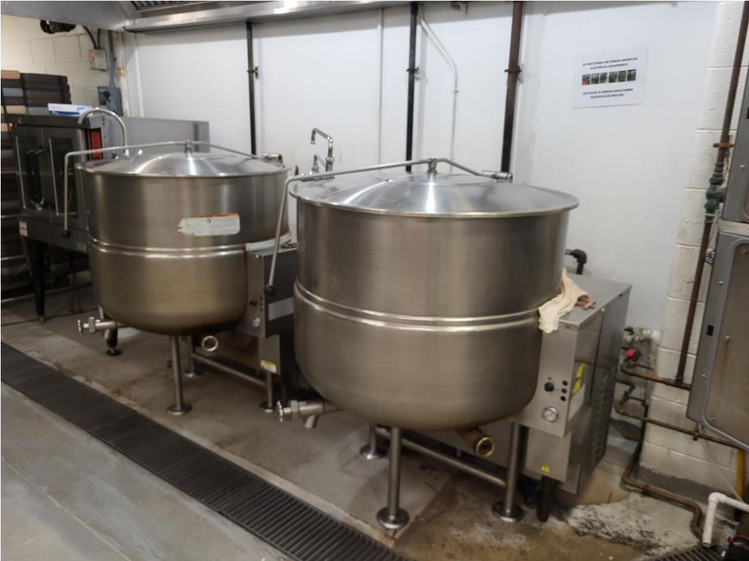
Installation area - view of current steam kettle equipment.
