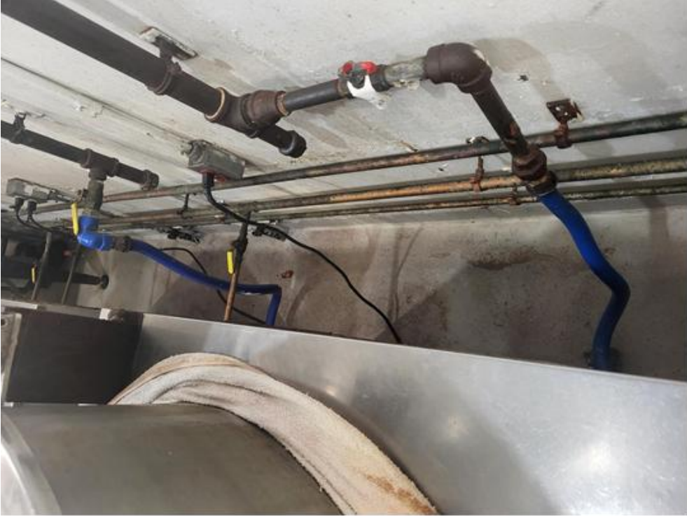
Installation area - view of clearance and hookups behind current steam kettle equipment.
